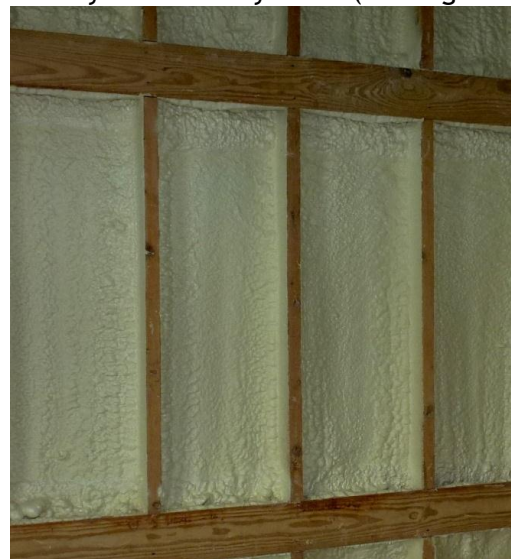
Figure 7: Space between interior finish and SPF due to partially filled wall cavity.
