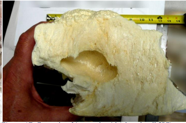
Figure 17: Example of internal void (closed-cell SPF).
