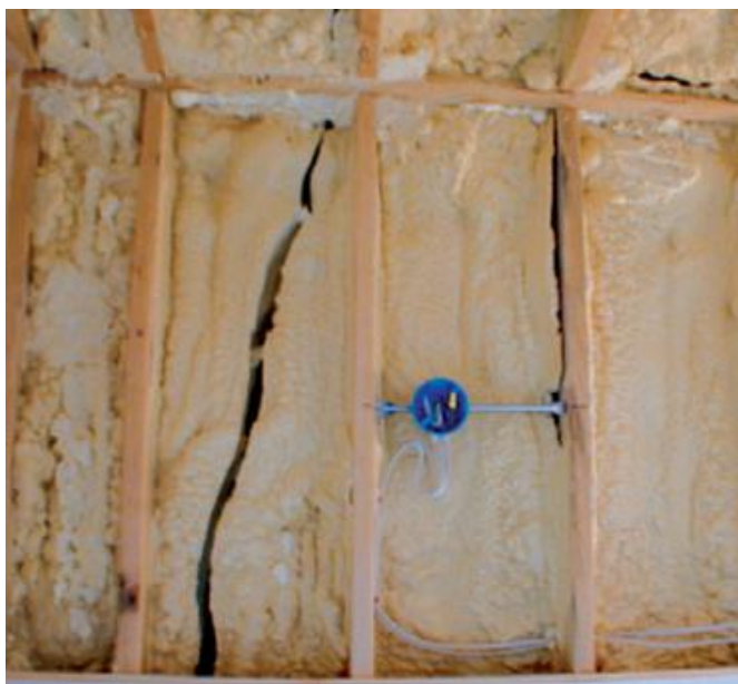
Figure 1: Crack in foam. (Photo courtesy of Henri Fennell Consulting)
