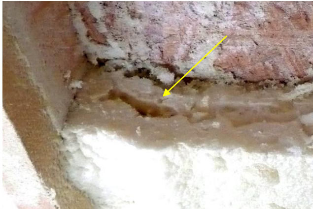
Figure 16: Example of internal void (open-cell SPF).
