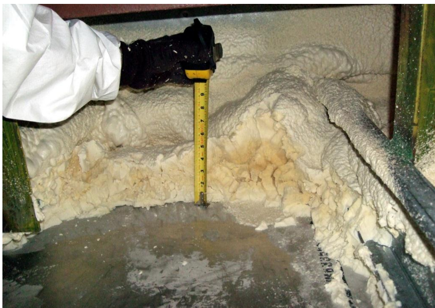
Figure 14: Scorching from applying too thick causing excessive heat.
