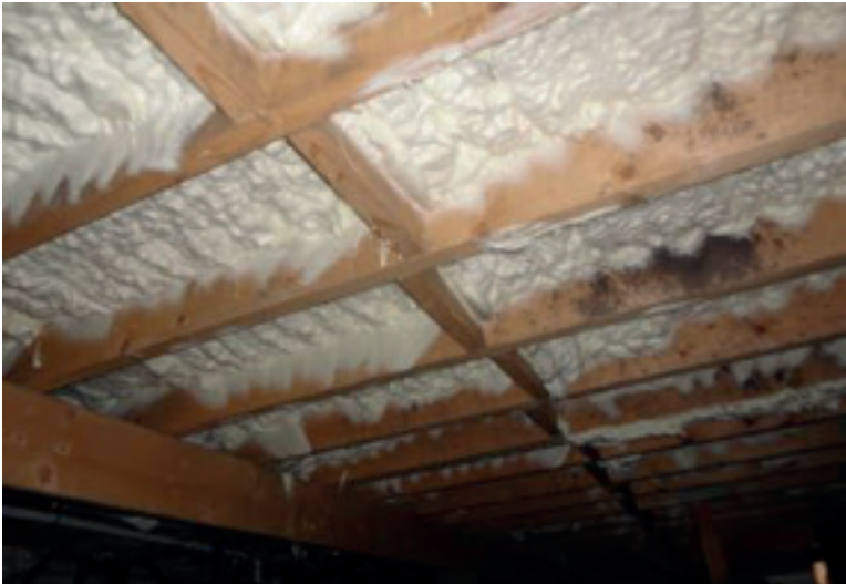
FIGURE 17. Installation of SPF below the subfloor allows complete access to the band joist and sill plate for inspection.
