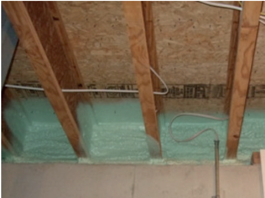
FIGURE 12. Closed-cell SPF insulation at the foundation-framing area
