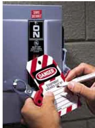
FIGURE 3 - Deactivate and mark HVAC system at electrical panel (use LOTO procedure and indicate date, time and name of person applying the tag).
