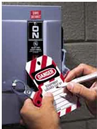
FIGURE 1: Deactivate and mark HVAC system at electrical panel (use LOTO procedure and indicate date, time and name of person applying the tag).
